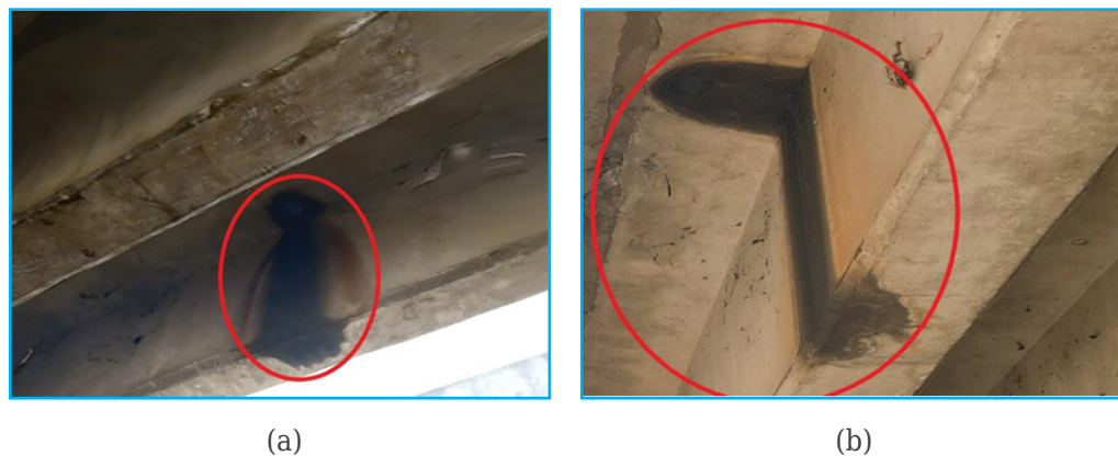
Figure 13. Identified deterioration caused by water: 3D reconstructed model (left) and the real image (right)
