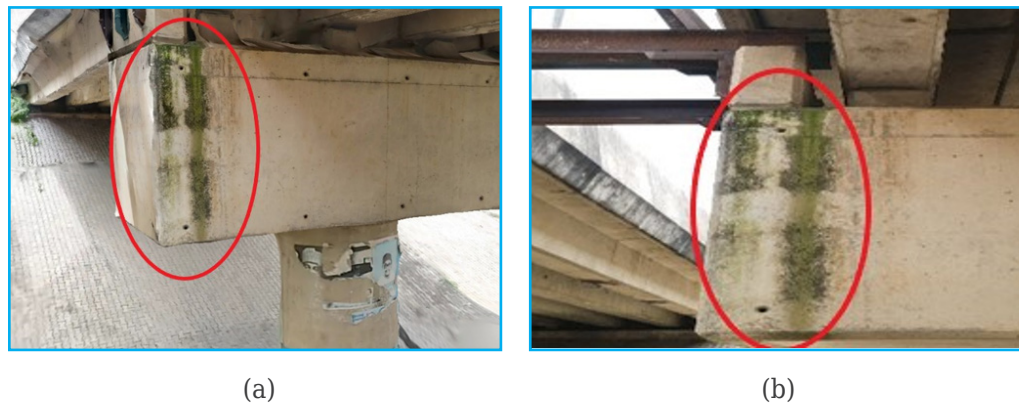
Figure 12. Identified damage due to algae: 3D reconstructed model (left) and the real image (right)
